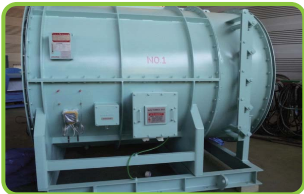
희석 fan(Dilution air fan)
